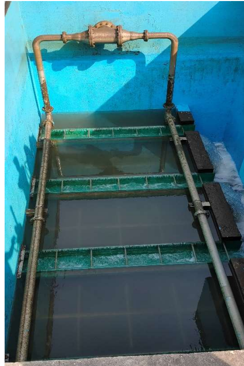
Clear water (completion of backwash)
