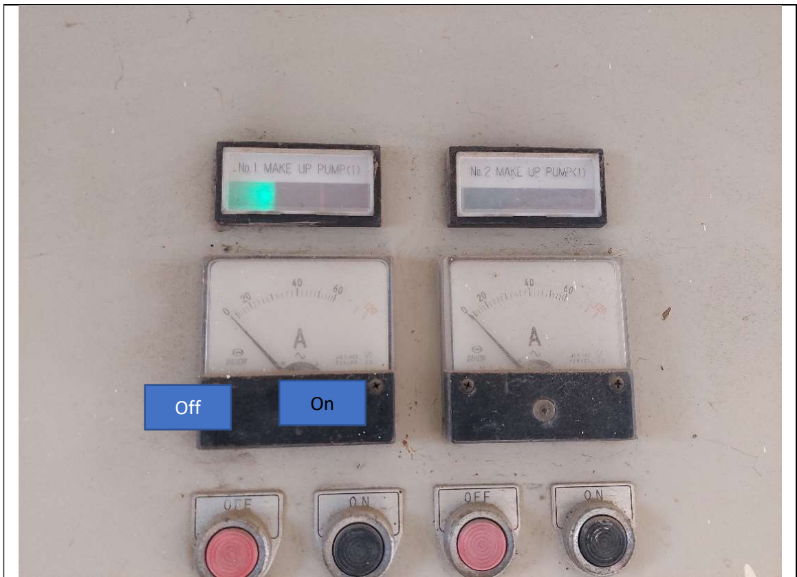
On-Off panel of makeup pumps
