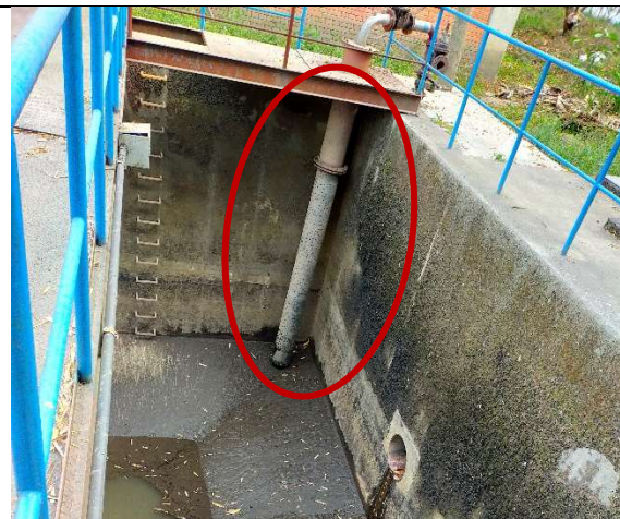
Suction pipe for recycling of sludge
