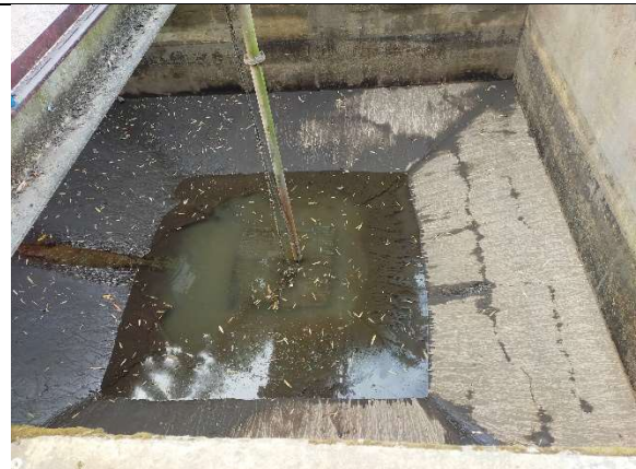
Sludge drainage basin (1 of 4)
