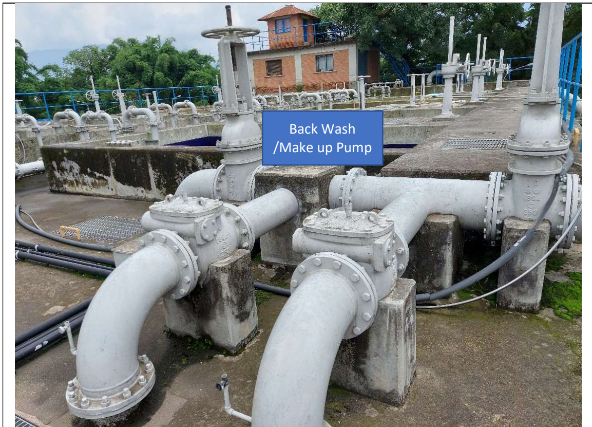
Backwash/ makeup pumps
