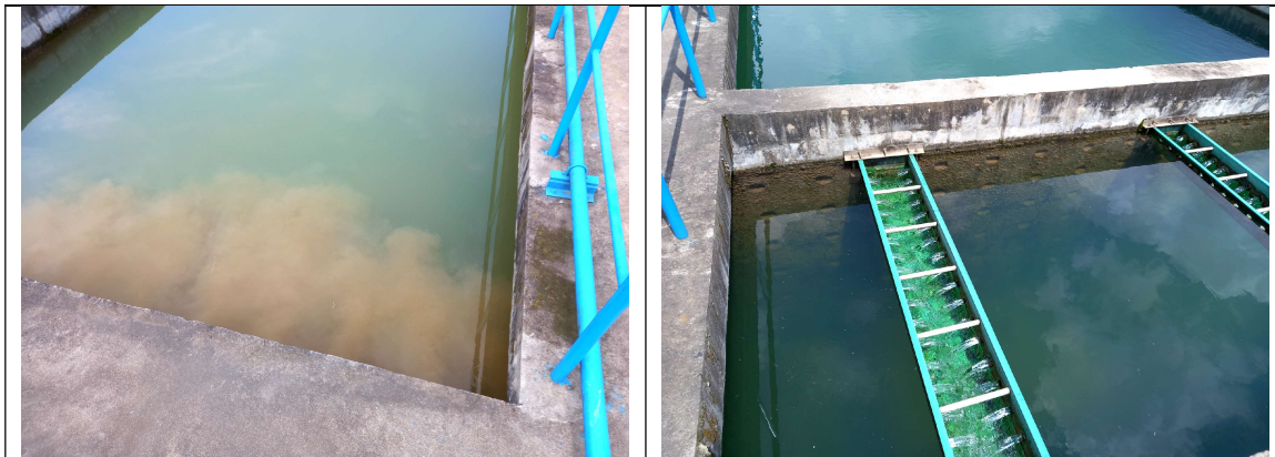
Inlet of Sedimentation Basin
