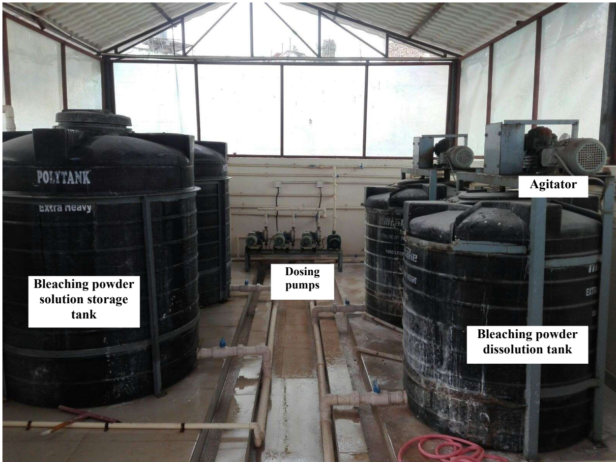
Photo 4: Bleaching powder dissolution and storage tanks in Bansbari WTP
