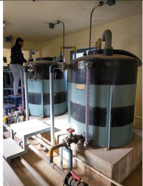
PAC solution storage tanks
