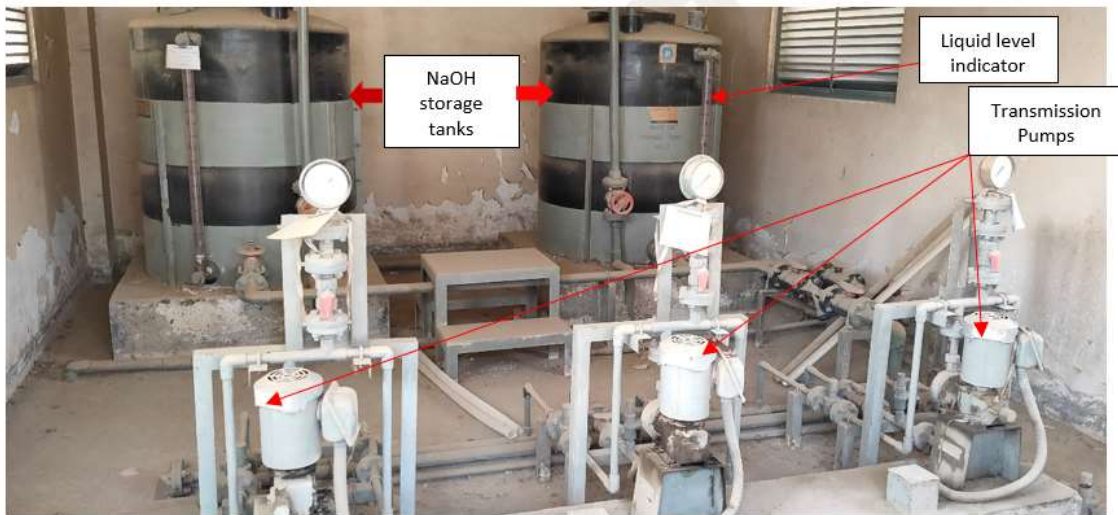
Figure 7: NaOH solution storage and feeding equipment
