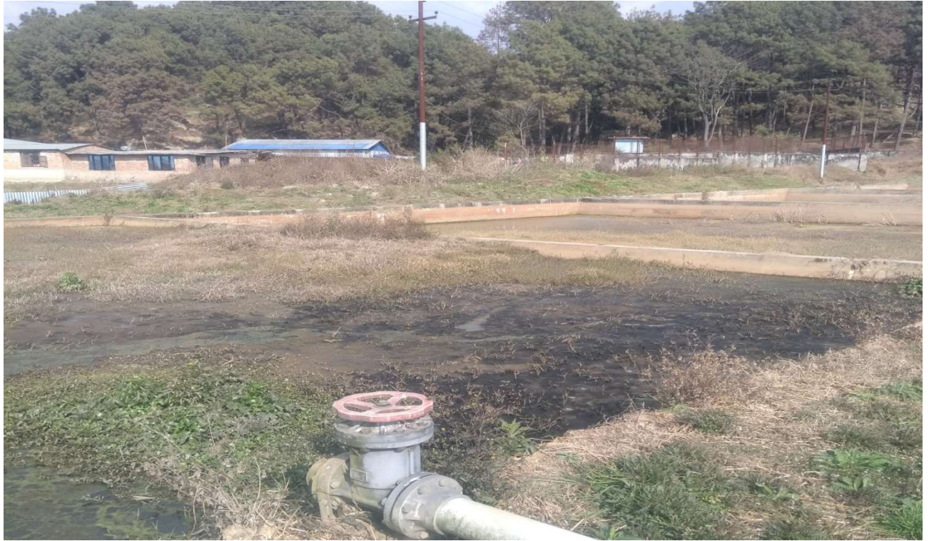
Figure 22: Sludge drying bed
