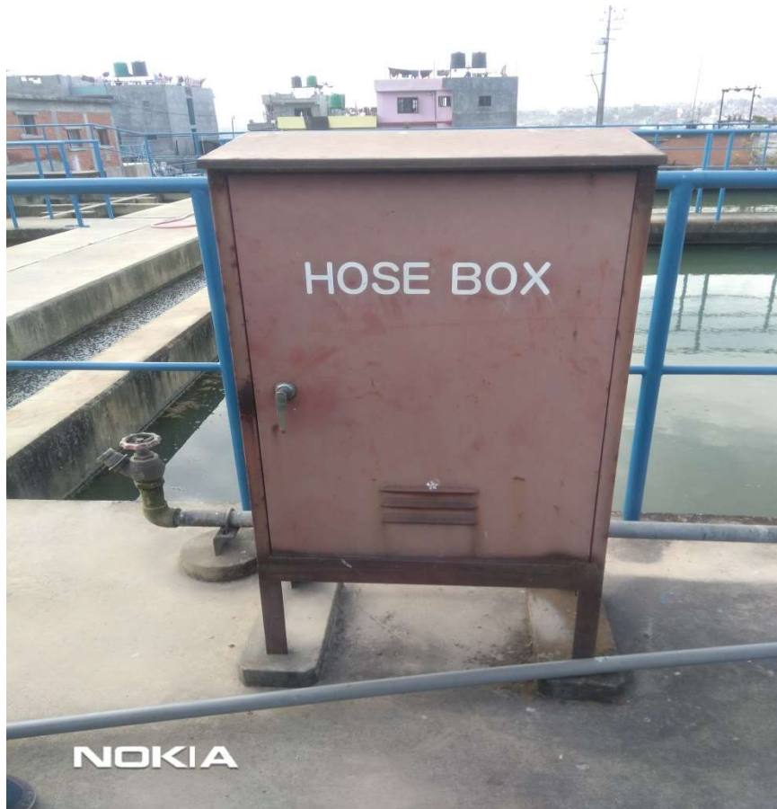
Figure 28: Hose box for washing
