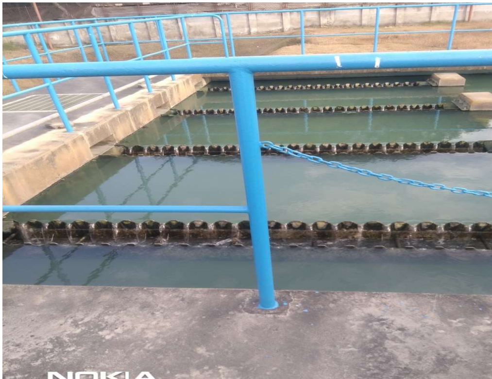
Figure 25: Sedimentation basin – Trough
