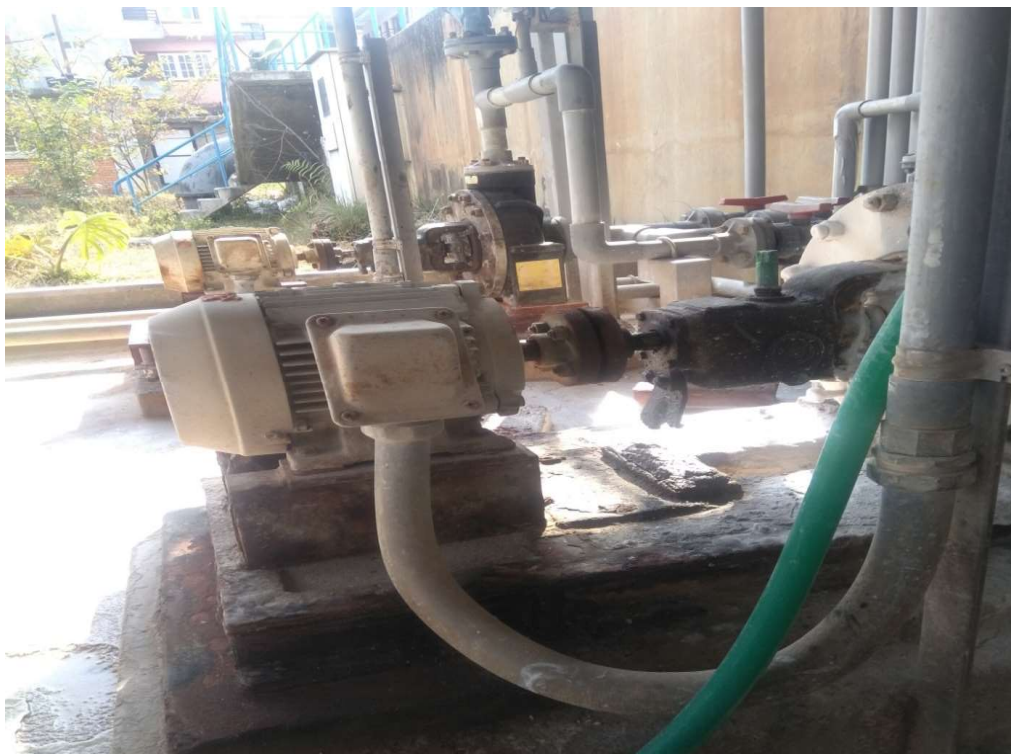
Figure 19: Chlorine Transfer pump
