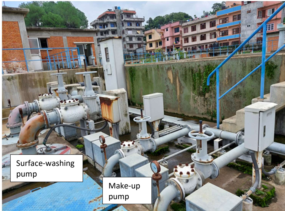
Figure 6: Pumps of rapid sand filter basins
