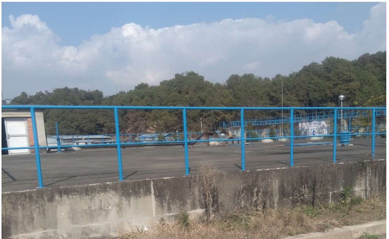
Figure 23: Clear water reservoir
