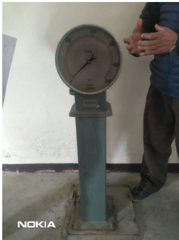
Figure 27:Raw water flow meter (not operational currently)
