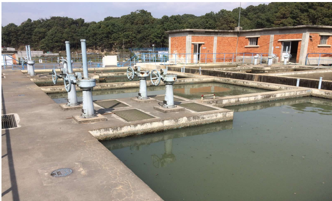
Figure 17: Rapid Sand Filter( Raw water gate and Raw water valve)
