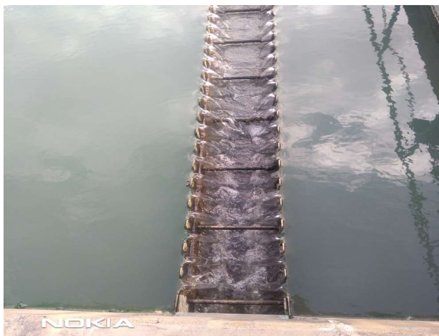
Figure 29: Sedimentation basin - trough
