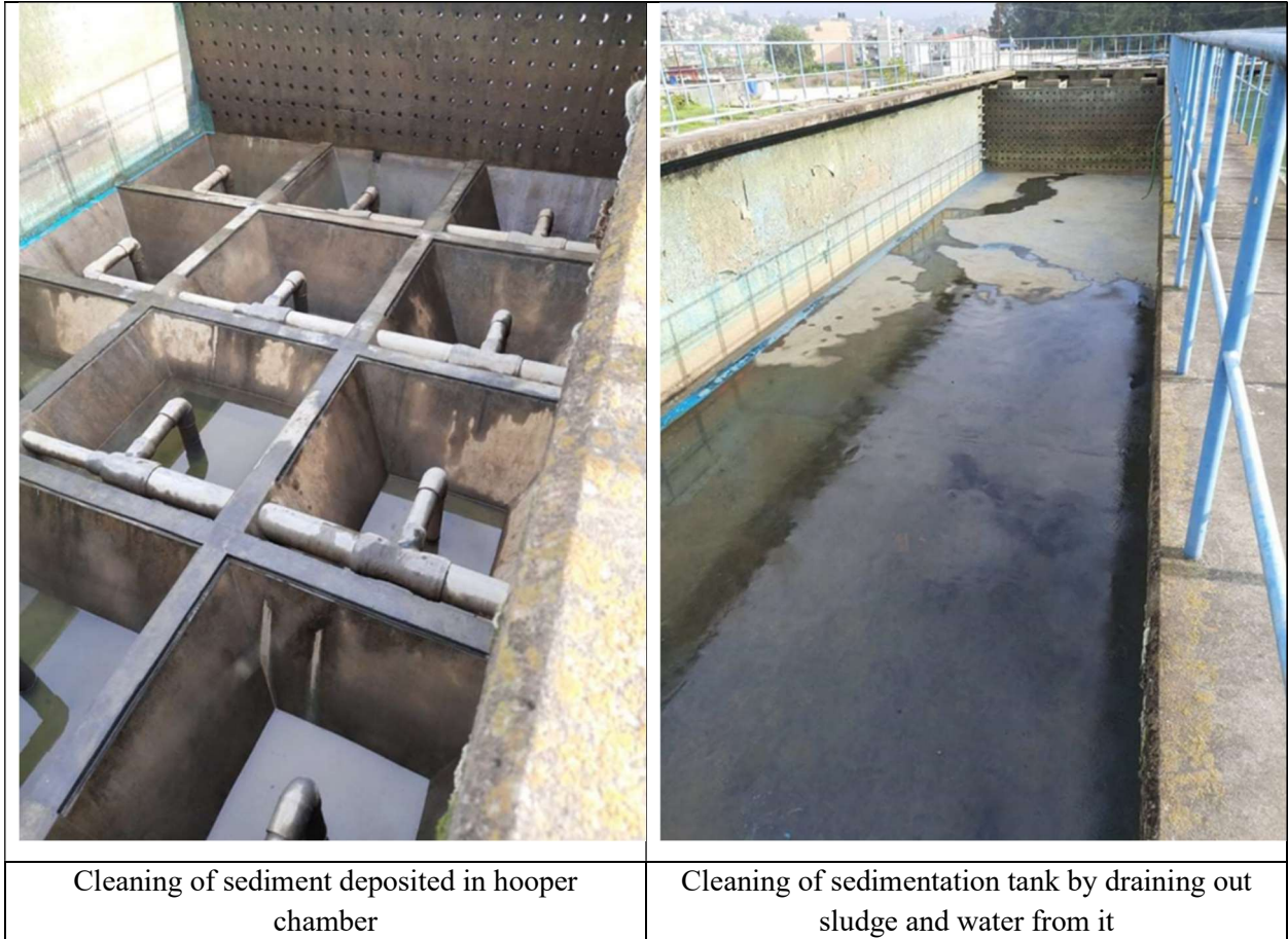
Figure 3: Sedimentation basin during draw-off and cleaning process
