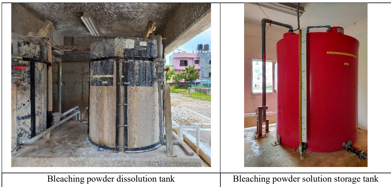
Photo 2: Bleaching powder dissolution and storage tanks in Bode WTP
