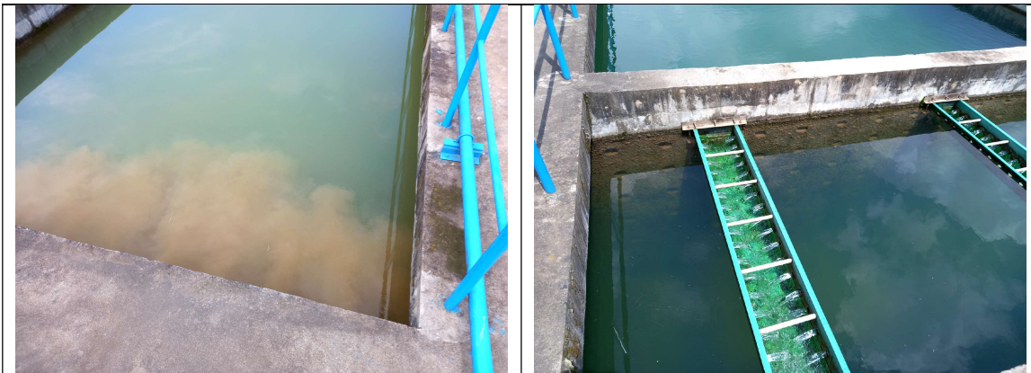
Inlet of Sedimentation Basin
