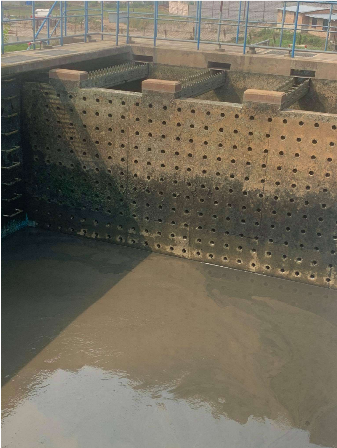
Figure 30: Sedimentation basin after draw-off during cleaning process
