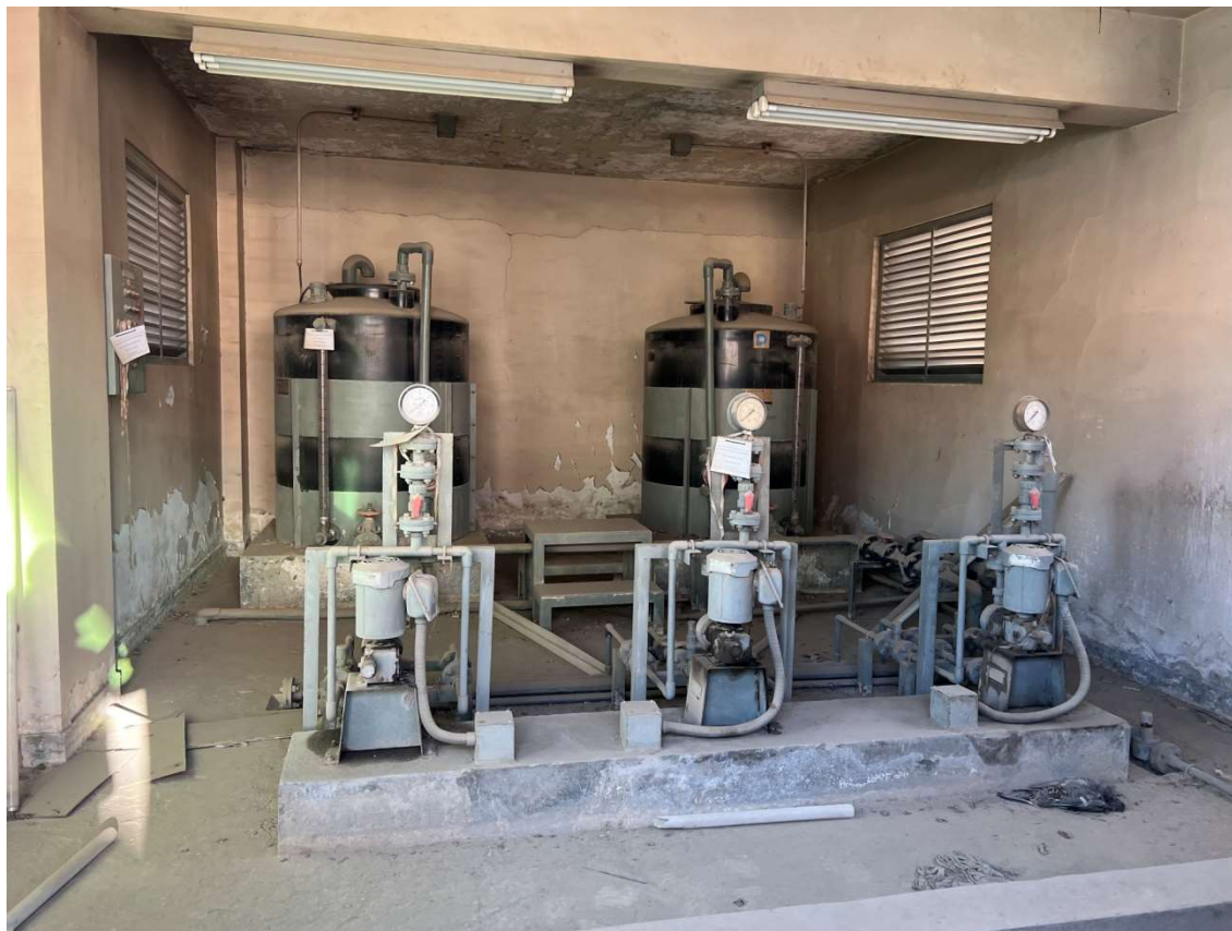
Figure 6: Caustic soda storage and feeding room
