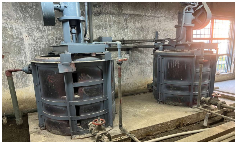
Figure 21: Lime dissolution tanks
