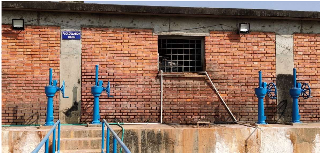
Figure 7: Valves and gates to regulate groundwater and surface water
