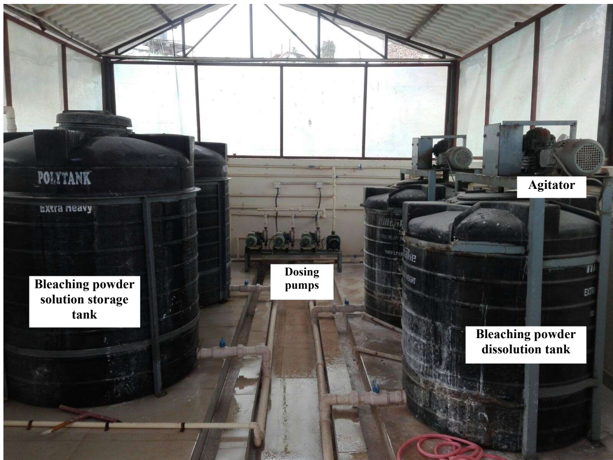
Photo 5: Bleaching powder dissolution and storage tanks in Mahankalchaur WTP
