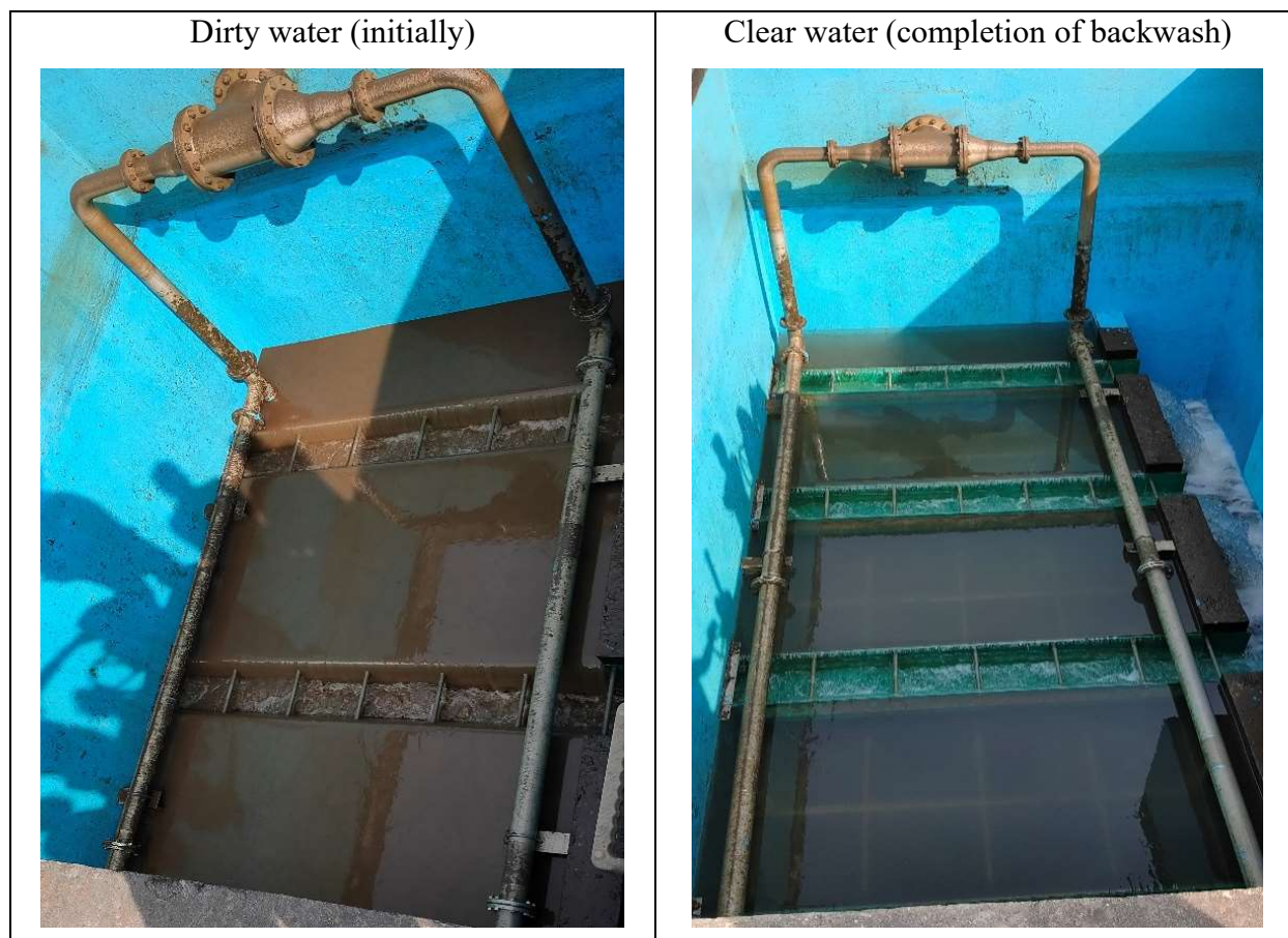
Figure 27: Condition of RSF bed level before and after backwash
