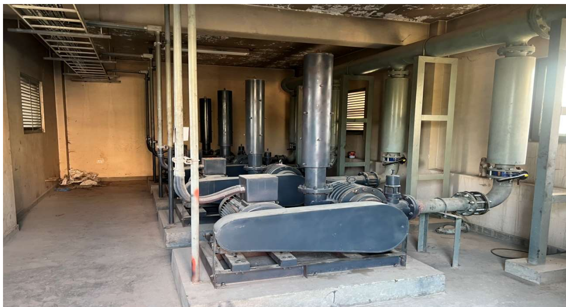
Figure 5: Air blower room
