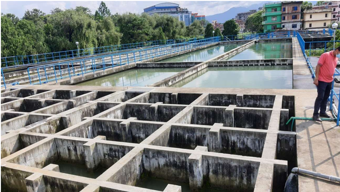
Figure 9: Flocculation and sedimentation basins
