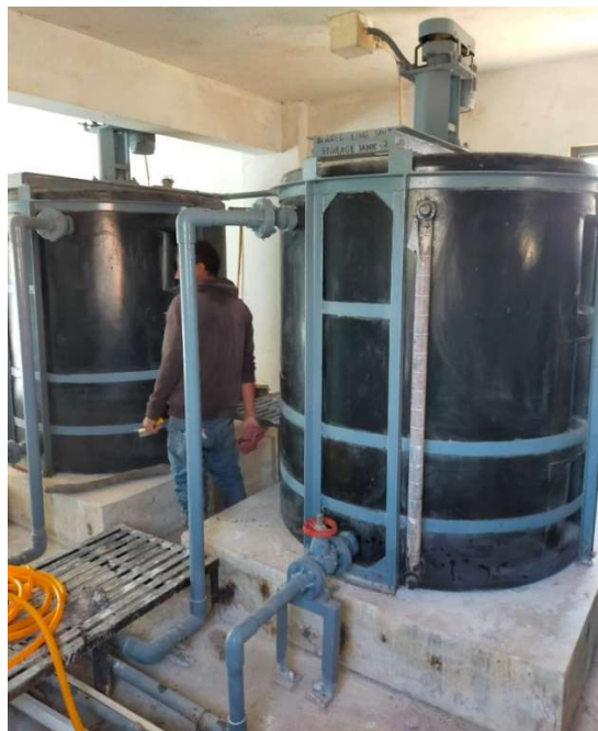
Figure 22: Lime solution storage tanks (2 Nos.)
