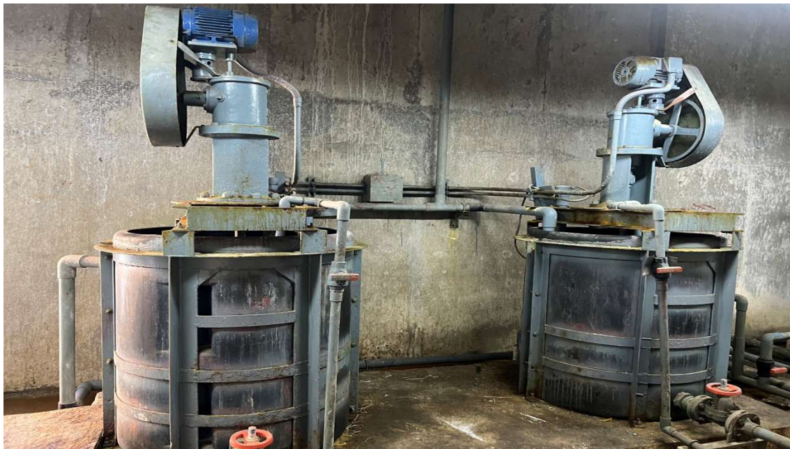
Figure 11: PAC dissolution tanks
