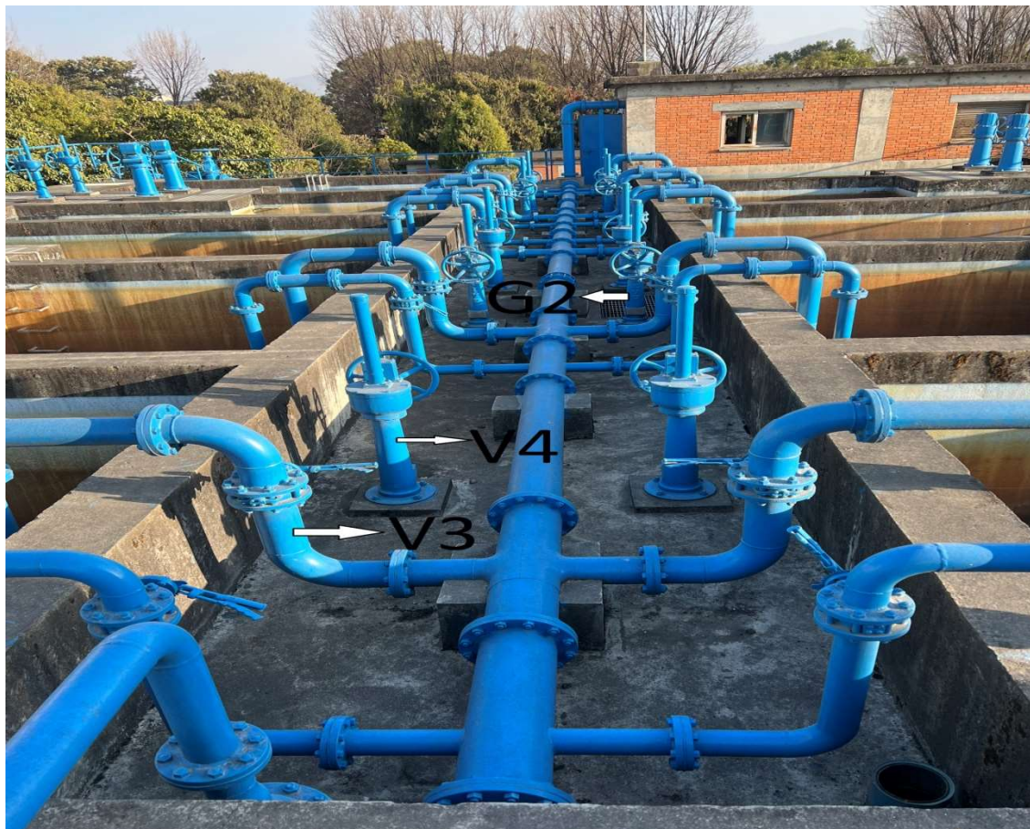
Figure 4: Air valve, backwash and water discharge valves
