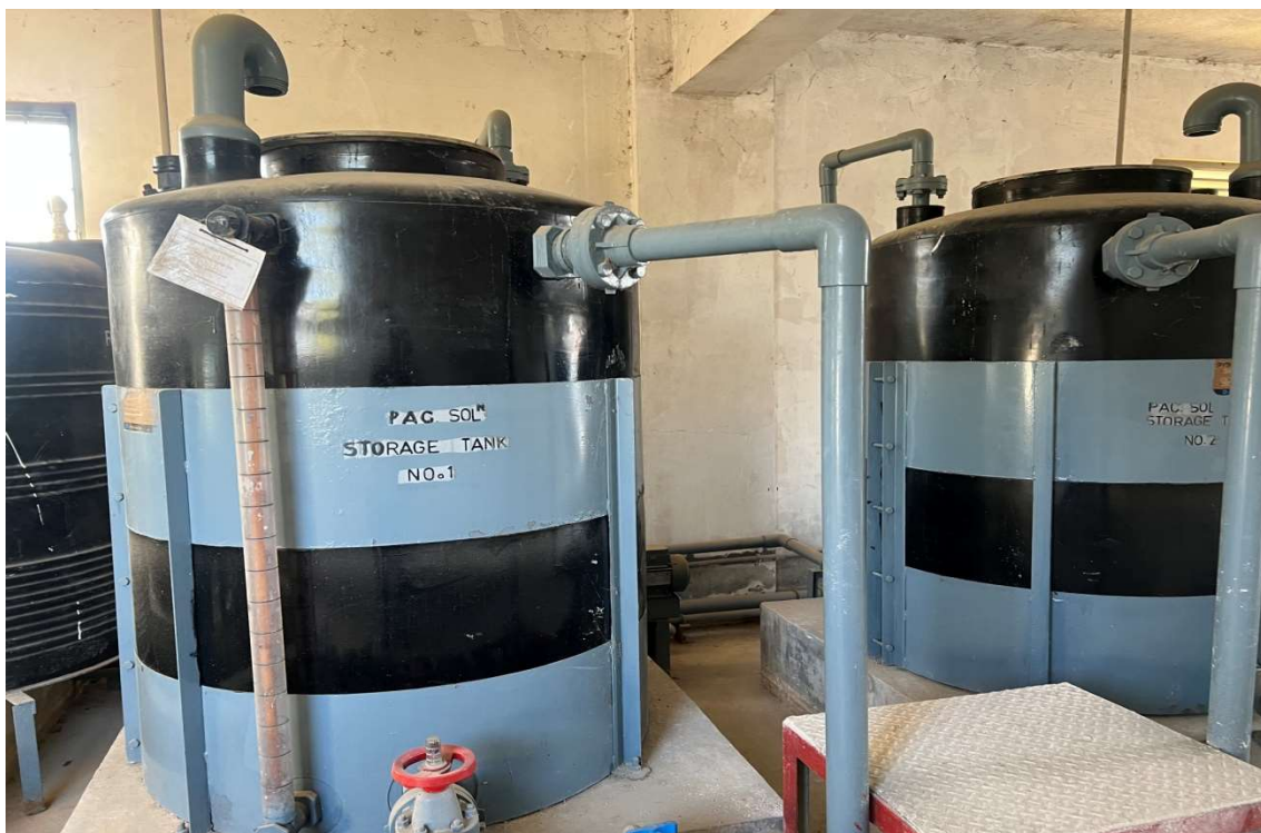
Figure 13: PAC solution storage tanks
