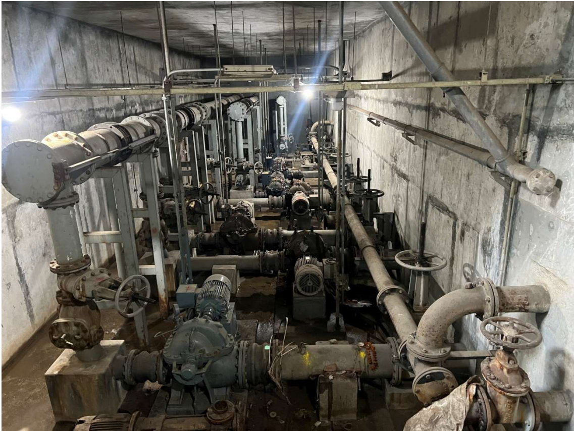
Figure 28: Transmission pumps and drainage pumps
