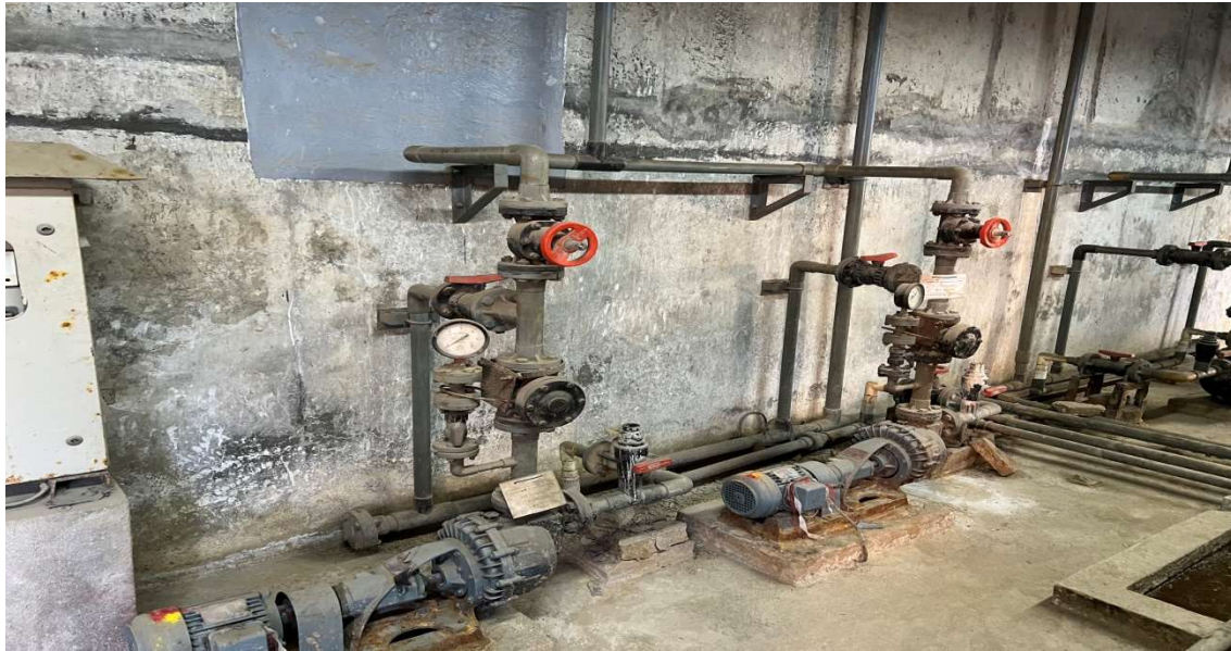
Figure 12: PAC solution shifting (transferring) pumps
