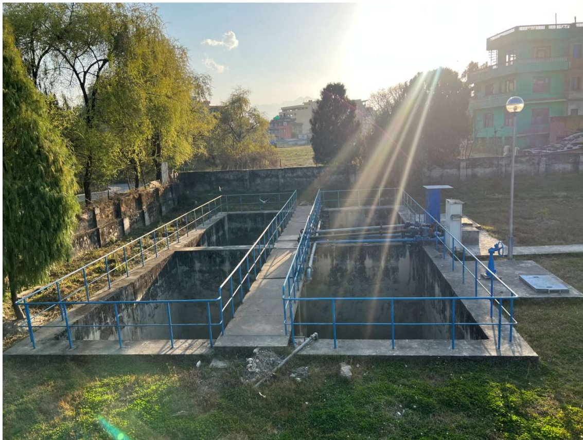
Figure 29: Sludge drainage basins
