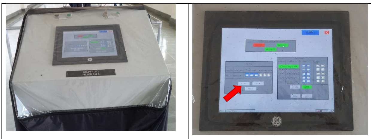
Photo 12: Local console panel of filters
