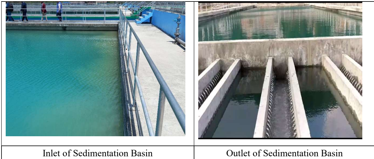
Photo 7: Floc formation at the inlet of Sedimentation basin (left) and outlet of Sedimentation basin
