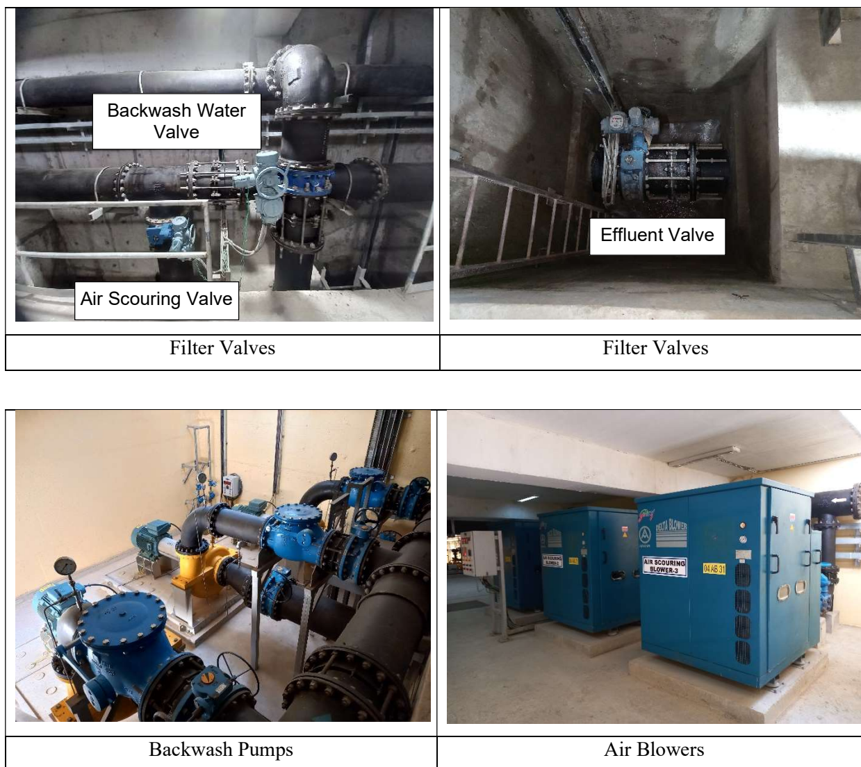
Photo 11: Filter equipment and facilities
