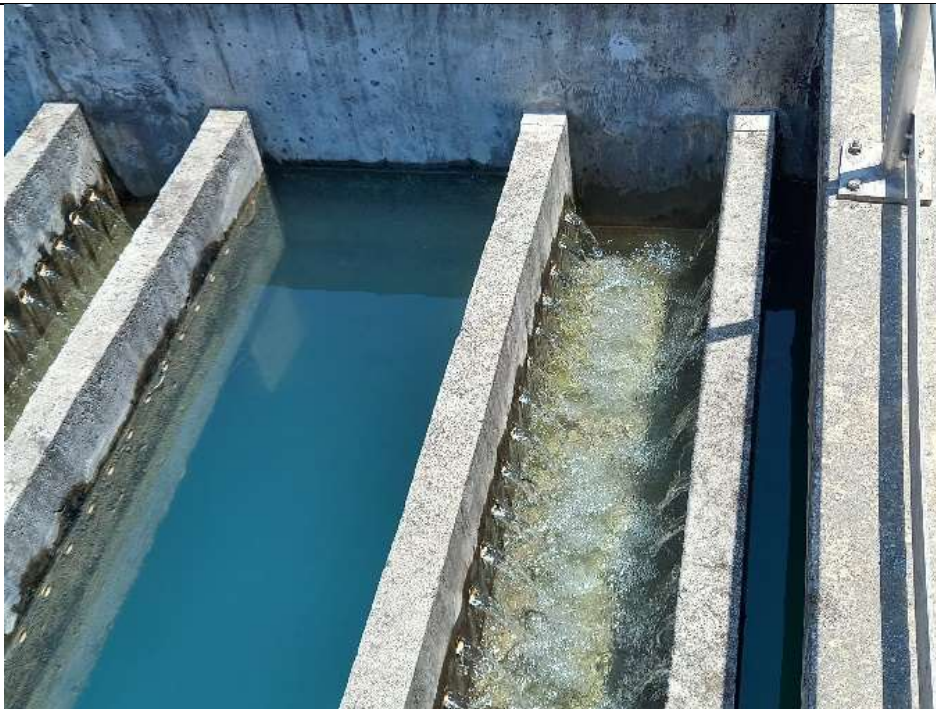
Outlet of Sedimentation Basin
