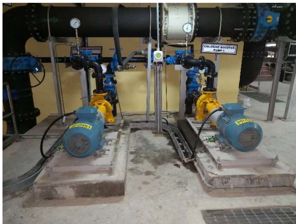
Photo 29: Chlorine Booster Pumps (Filter Gallery)
