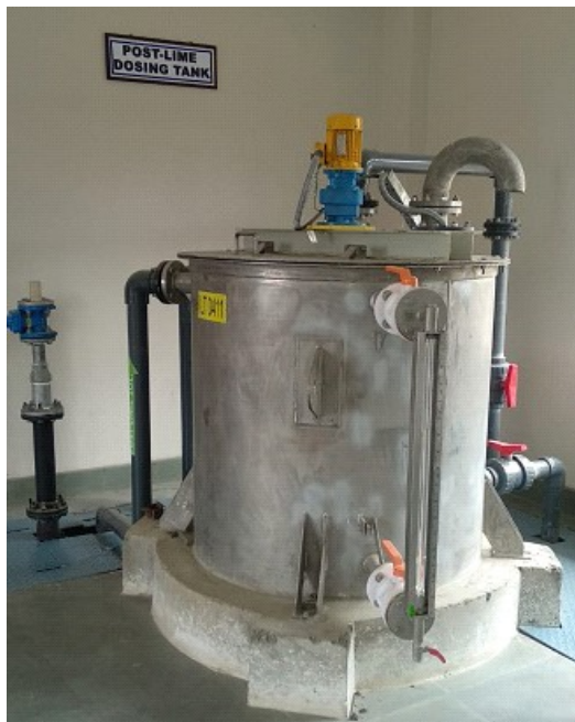
Post-lime dosing tank
