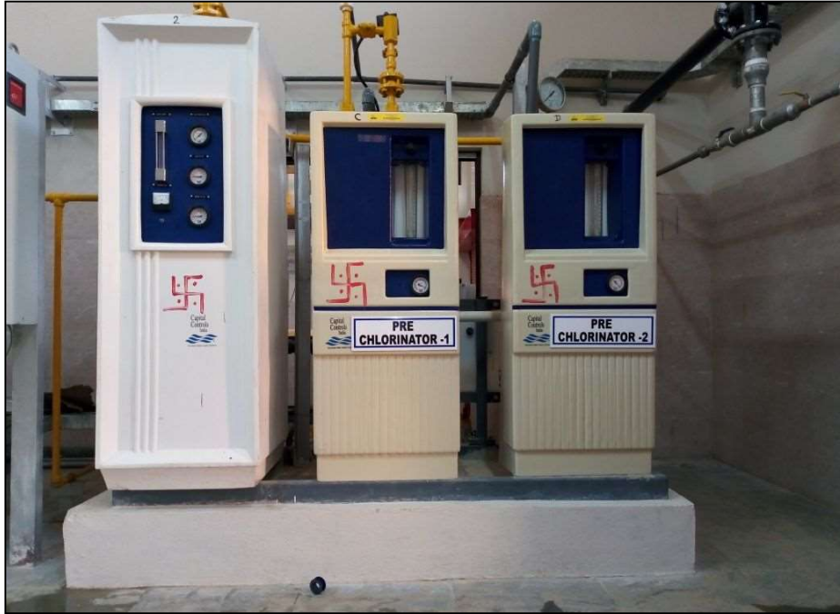
Photo 27: Chlorine Evaporators and Chlorinators
