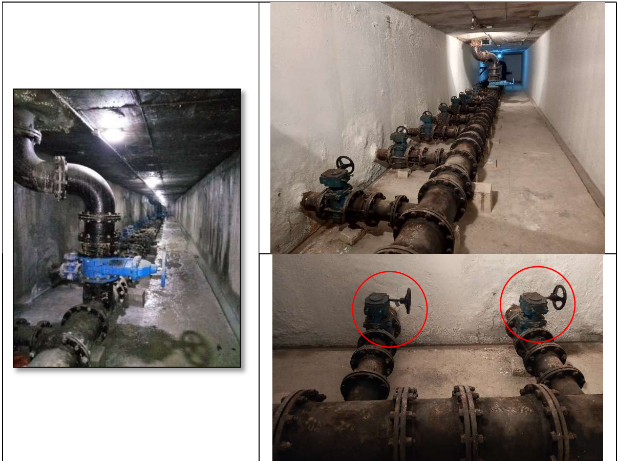
Photo 8: Sludge draining (desludging) valves of coagulation and sedimentation tanks
