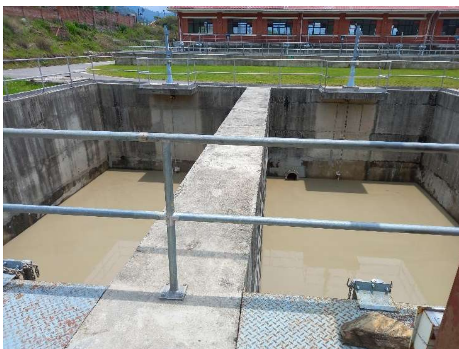
Photo 32: Backwash Water Recovery System
