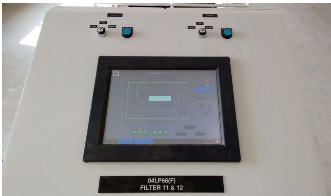
Photo 17: Filter’s local console and panel screens
