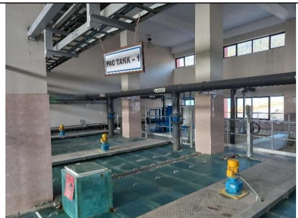
PAC Mixing Tanks
