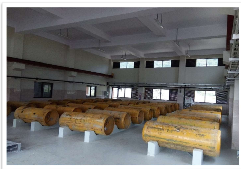
Photo 31: Chlorine Tonners Storage bay
